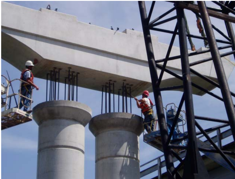
Figure 3.7 Connections with a Large Number of Connectors Require Larger Construction Tolerances (Lake Belton Bridge)
