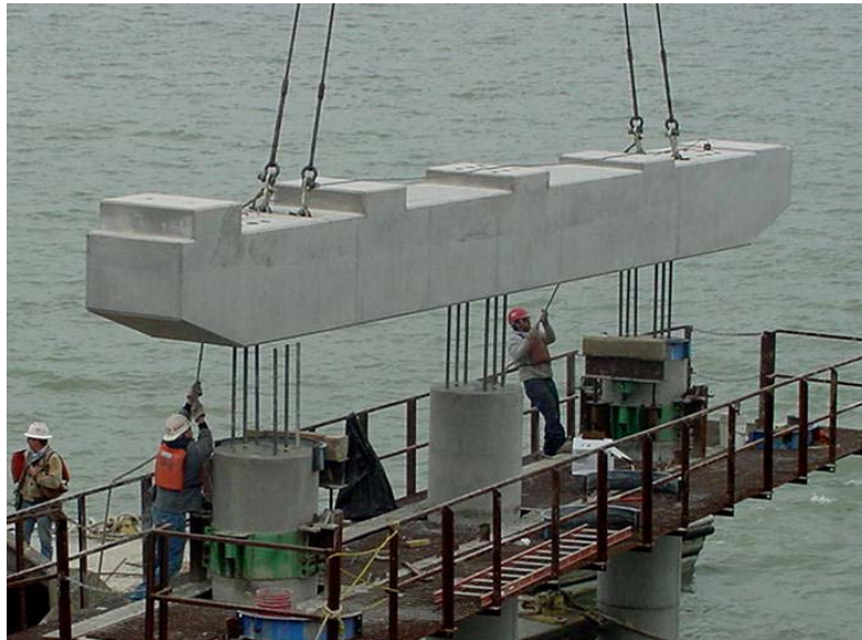
Figure 3.20 Precast Bent Cap Placement over Bridge Pier and Connectors (Lake Ray Hubbard Bridge)
