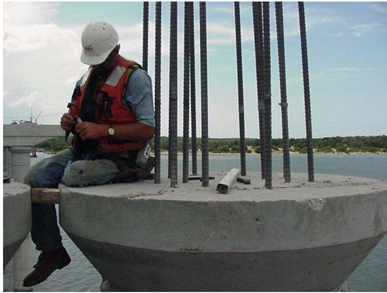
Figure 3.5 Improper Alignment of Reinforcing Bars that Project from Bridge Column at Lake Belton Bridge Project
